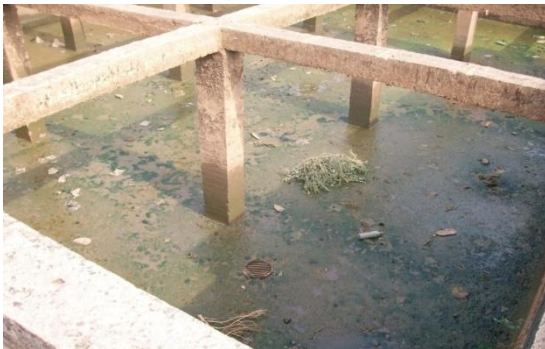
Plate1.1: The inside view of the injection well in military hospital
