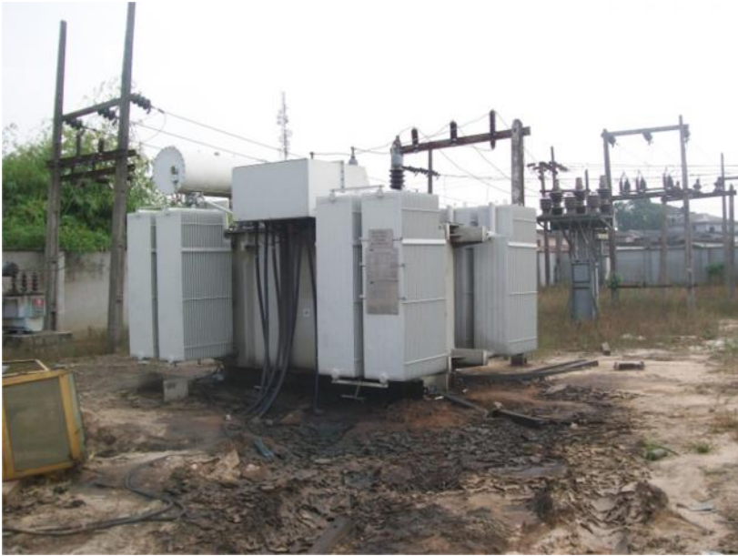
Fig 1: Otovwodo, 15MVA, 33/11KV Injection Substation.
