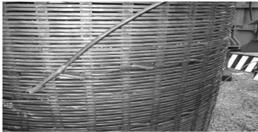
Figure 1: Paper insulated coil of a detanked transformer (Source: [18])
