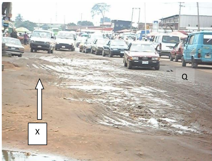
Figure 4: Failed portion in a road segment. Observe the effect of failed portion of road segment: Note that the vehicle marked Q has free space in front. Observe that the vehicle marked X is driving against traffic.
