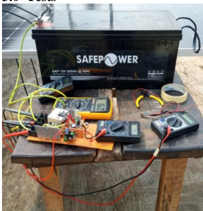
Figure 12: Test set-up of the charge controller circuit
